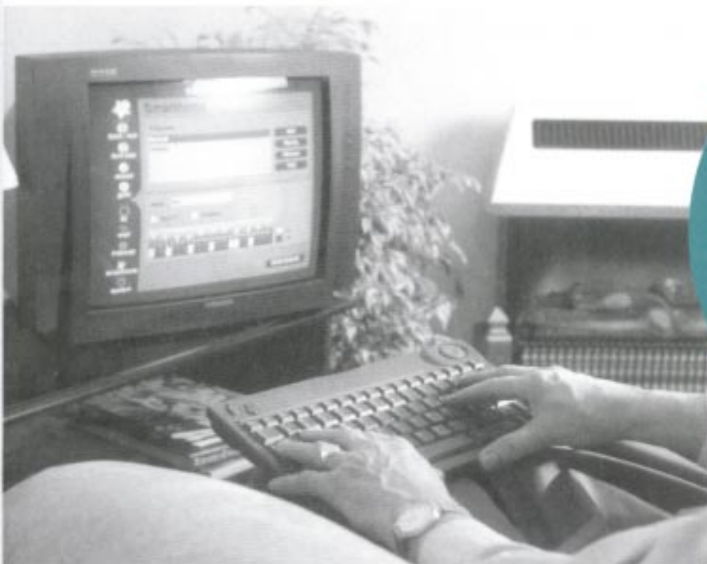
Using smart controls in the Joseph Rowntree Housing Trust house in York.
