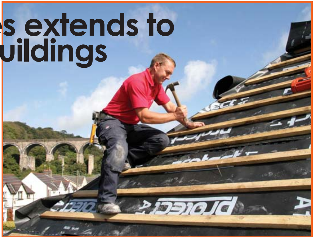
Re-roofing being undertaken by Ocean Housing Group, who trialled XB on two estates.
